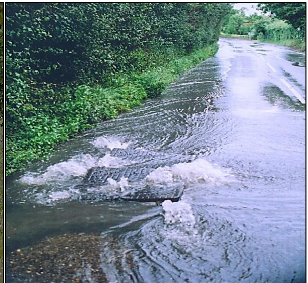
Figure 2 Manholes near The Hautboy, Ockham
