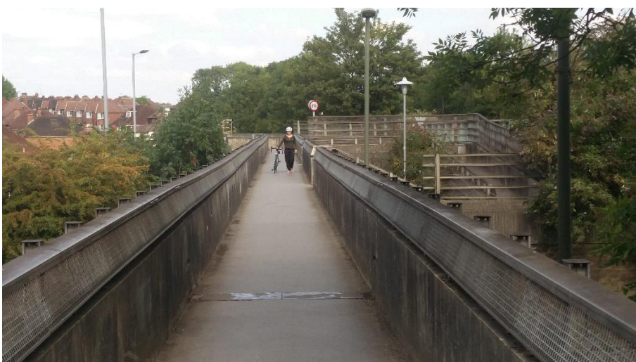
Wooden Bridge – main bridge over A3, showing narrow deck and low balustrades
