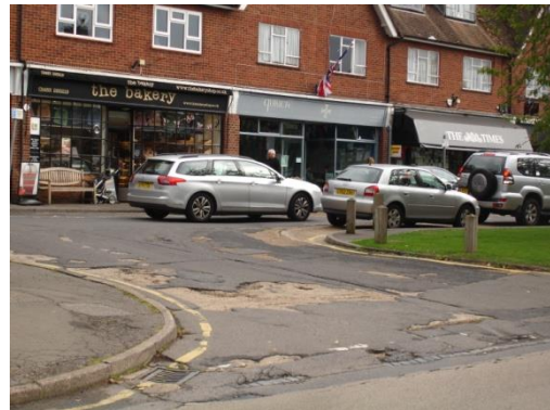
Degraded roadway into the central part of Station Parade.
